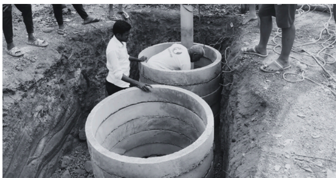
Dhanushi Bore well recharge
